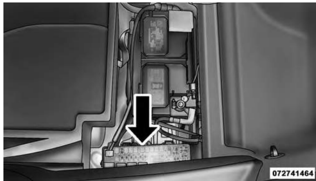
Rear Power Distribution Center
